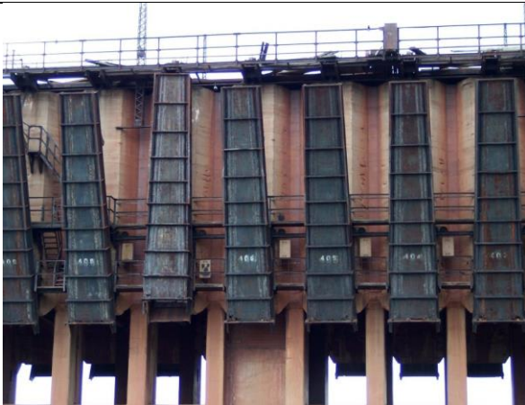
Close-up of the ore chutes on the last remaining ore dock in Ashland, Wisconsin. It was built in 1916. The superstructure was demolished in 2013 so that the base can be converted to a park. (Author photo)
